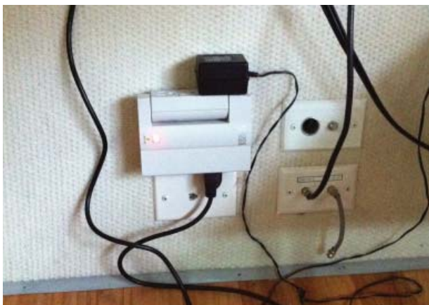
AC/DC CONVERTER BOX
